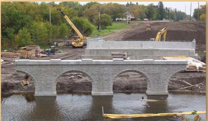
East pier prior to stain application
